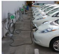
Electrification of Transportation
