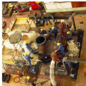
Power Supply & Generation
