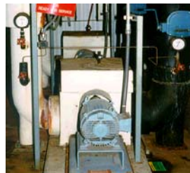
Pump head: 36 m Flow rate: 97.6 m 3 /h => hydraulic power: 9.6 kW Combined pump and motor efficiency = 59%
