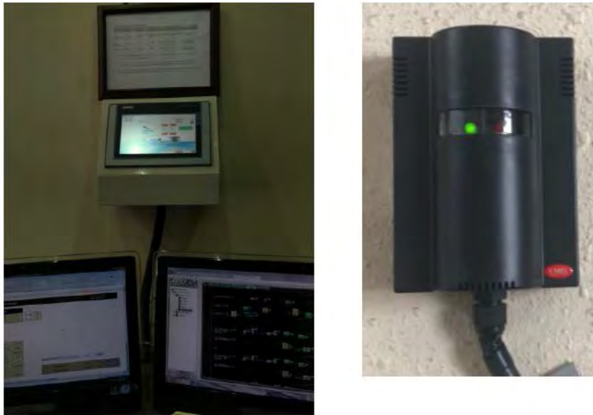
Figure 3.1: Control Alarm Panel and HC-290 sensors
