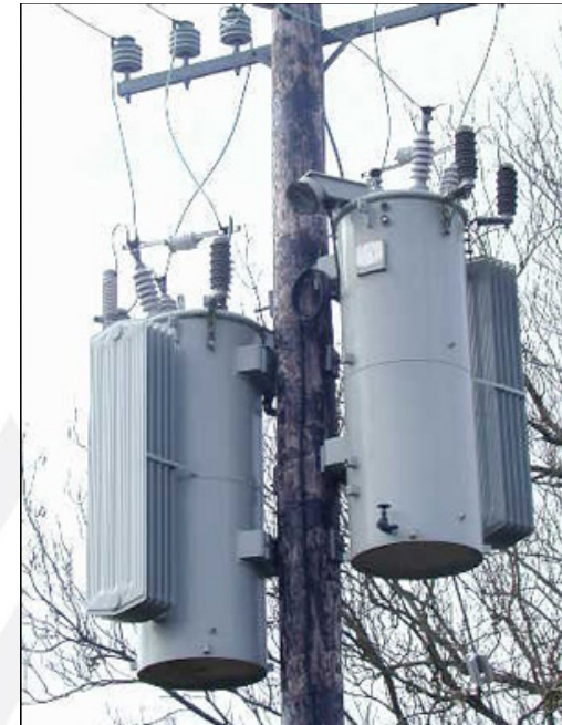
2 Single Phase Voltage Regulators
