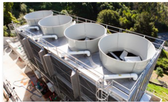
LBNL Compressorless Cooling
