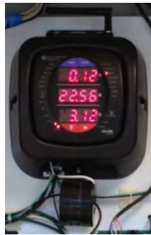
Figure 38 Three phase digital power meter with external current transformer
