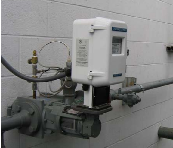
Figure 8: Digital Gas Meter Required for DER Systems by SDG&E
