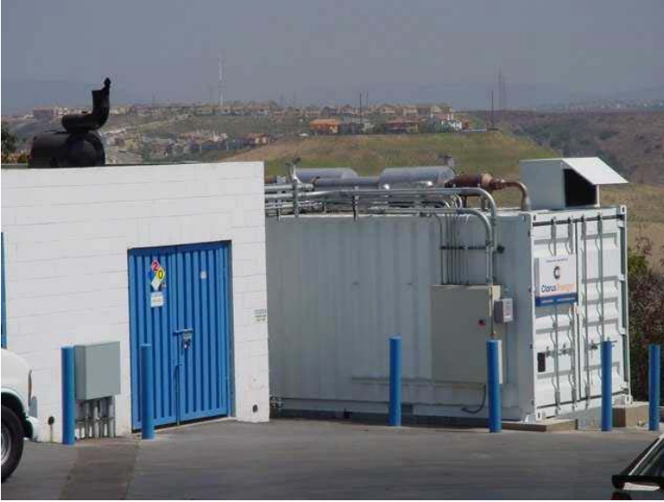
Figure 26: Generators in Place
