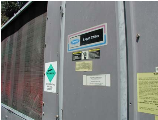
Figure 7: The Electric Chiller
