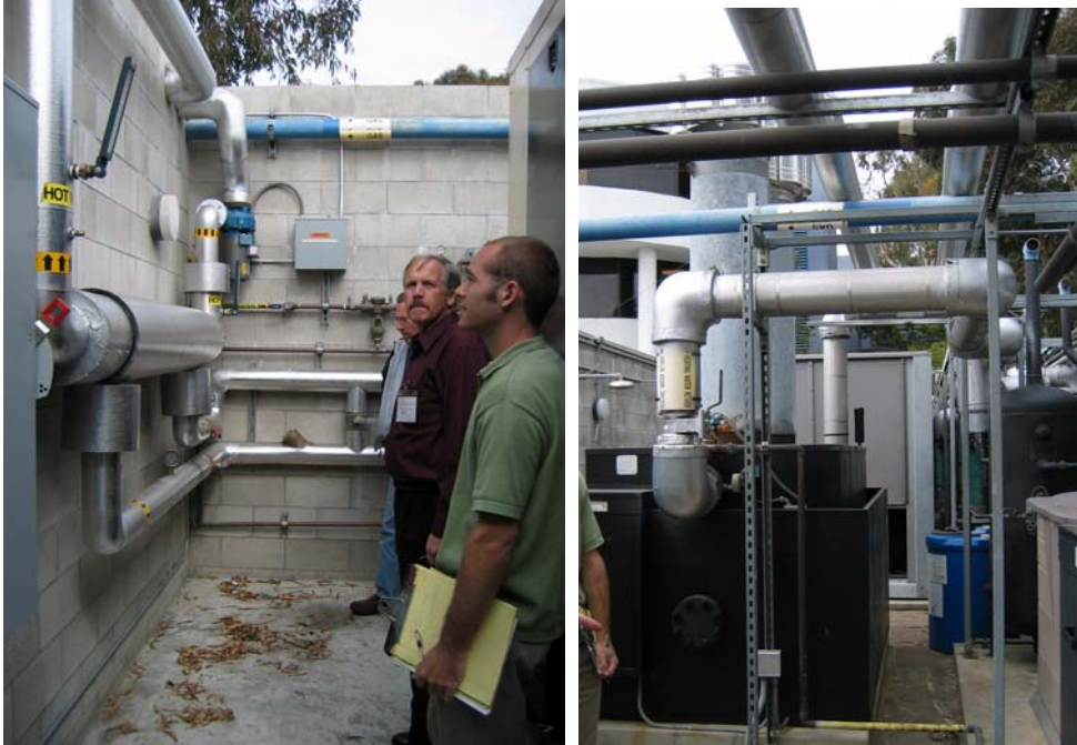
Figure 6: Heat Exchanger (left) and Boiler and Building Hot-Water Loop (right)
