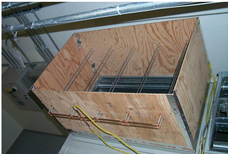
Figure II-4. An installed return flow grid assembly.
