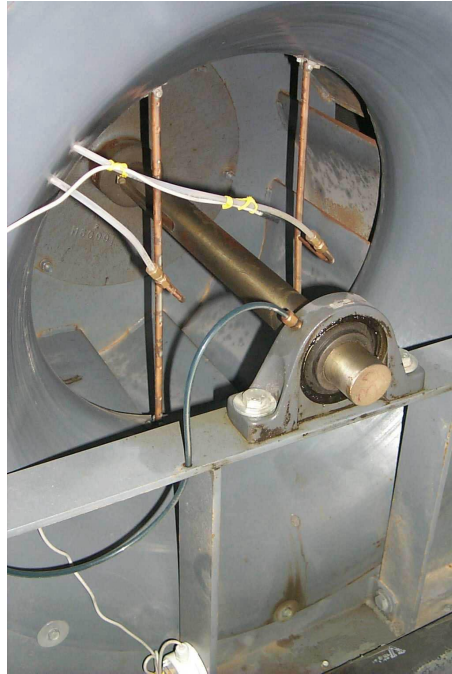
Figure II-2. Air-handler supply fan inlet. Note the two vertical copper tubes that comprise the airflow station. A tube for lubricating the shaft bearing can also be seen, as well as one of the temperature sensors that we installed.
