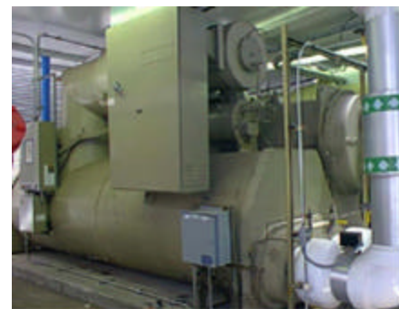
Figure 9. A typical chiller.
