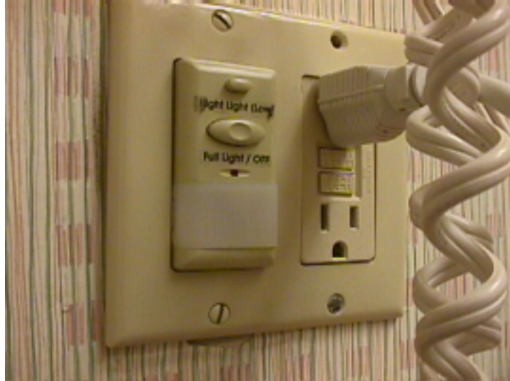
Figure 3: Bathroom controls were co-designed by LBNL and Wattstopper that utilized an occupancy sensor and a low-level “night light” feature.
