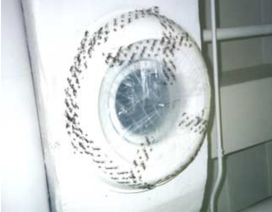
Figure 3. Sealed diffuser in Building LS-2
