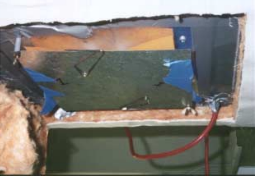
Figure 6. Impaction plate installed in Building LS-2
