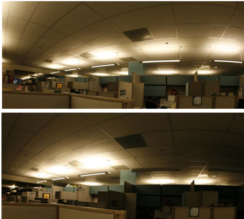
Figure 18: View of the ceiling with all nearby luminaires turned on (above) and with several luminaires turned off (below).
