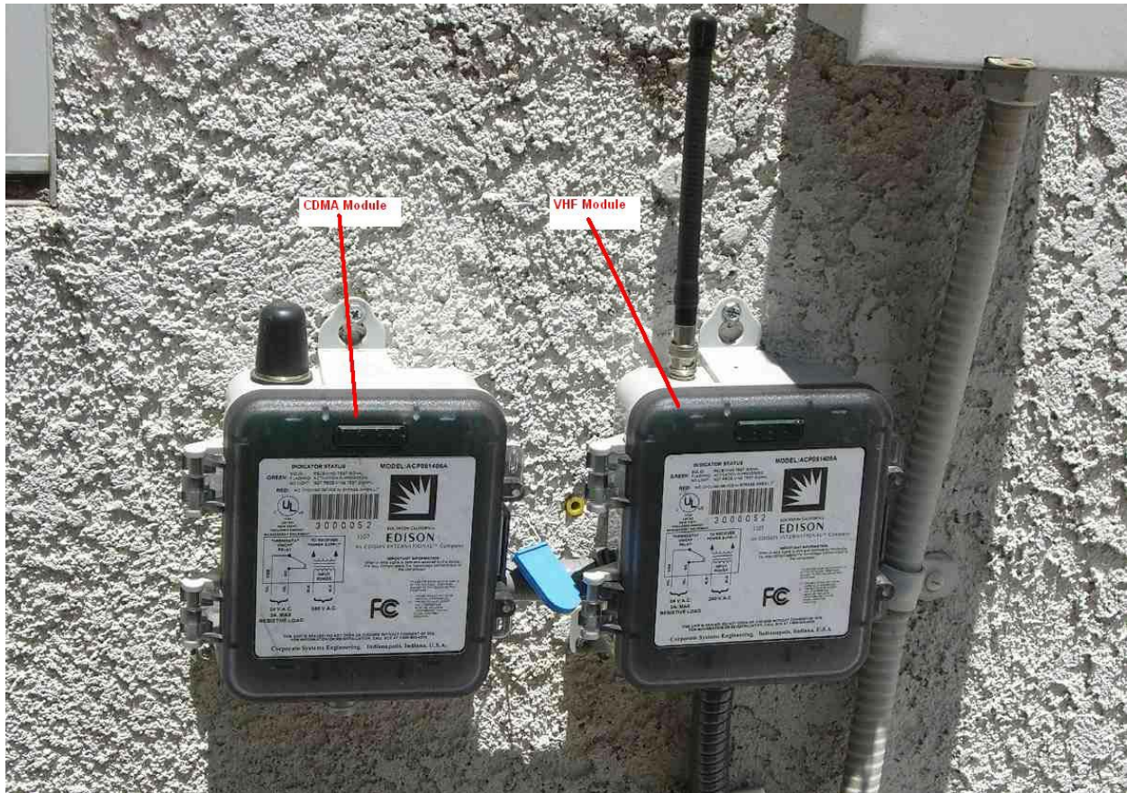
Figure 3.4 SCE AC Load Control Switch
