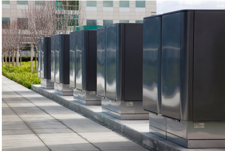
Figure 20. Bloom Energy fuel-cell power system
