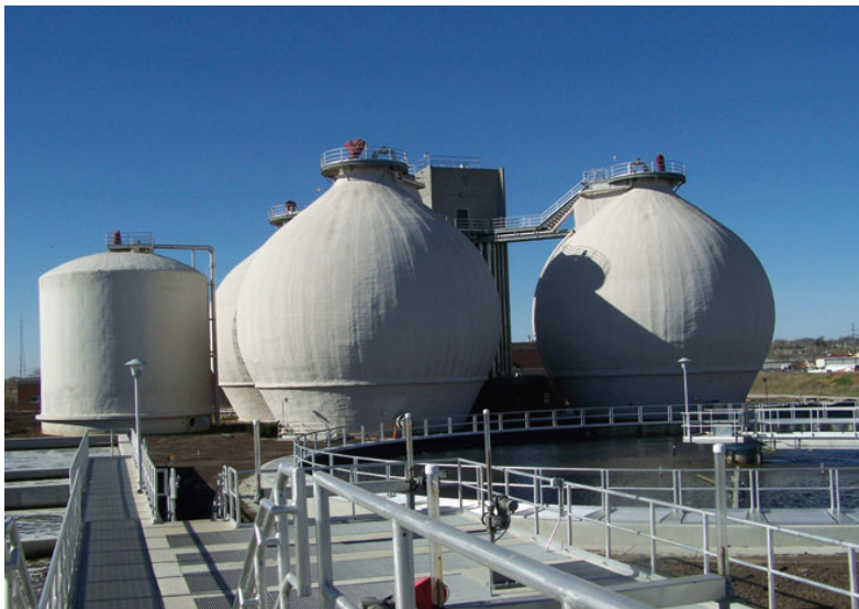
Figure 38. Anaerobic digesters at a wastewater treatment facility
