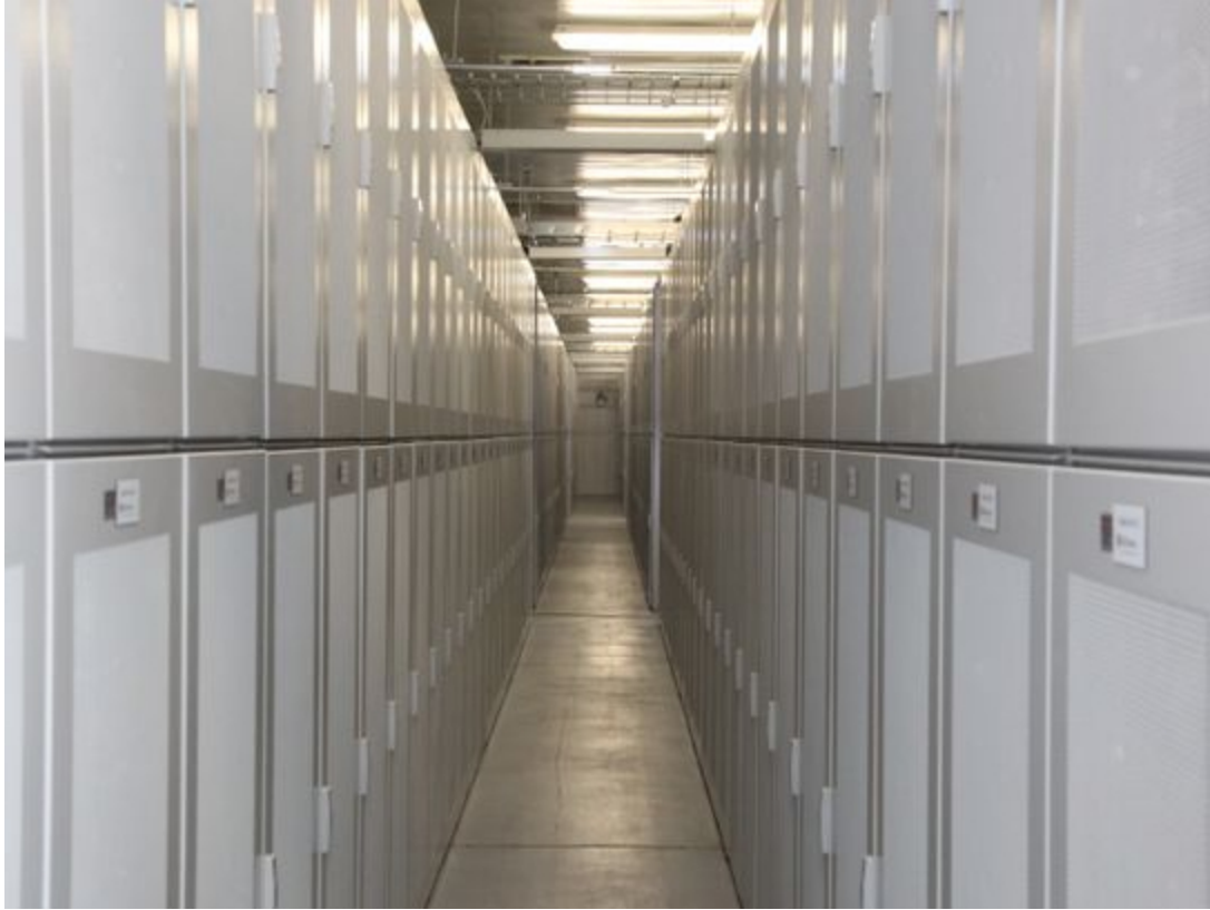
Figure 22. A 32-megawatt-hour lithium-ion energy storage project at the Monolith substation in the Tehachapi Mountains of California, USA
