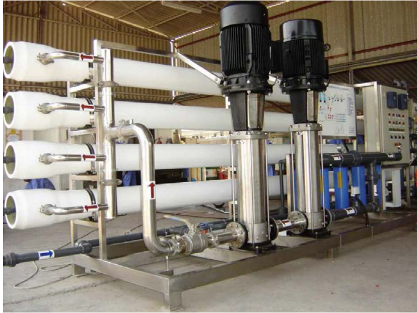
Figure 36. Reverse osmosis equipment at an industrial facility
