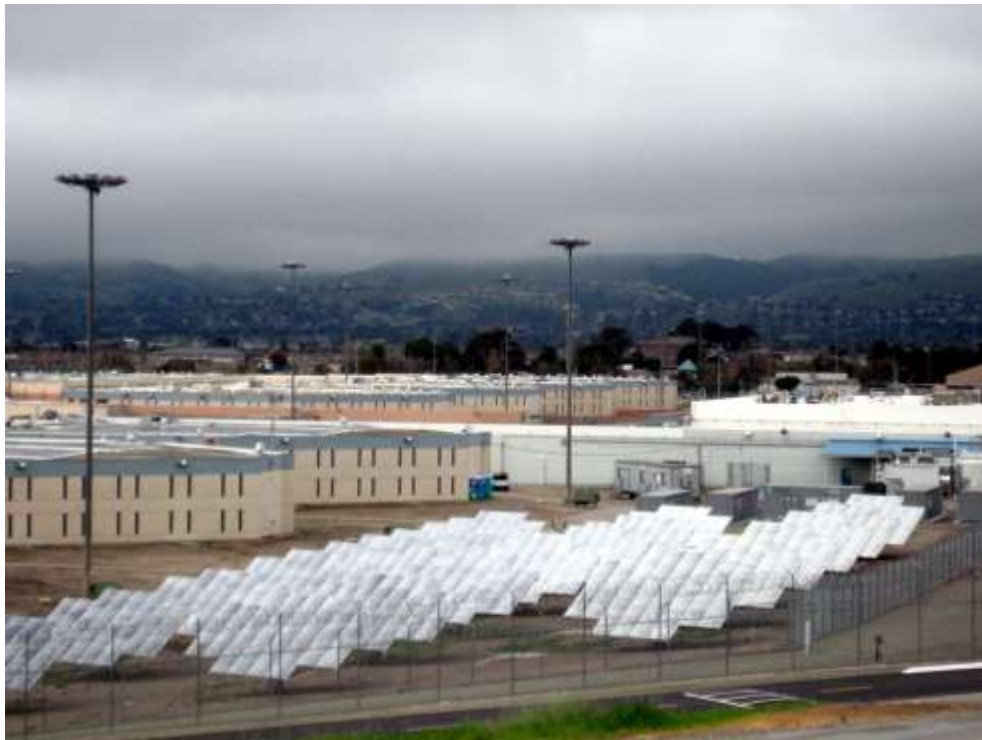
Figure 17: Recent photo of Santa Rita jail with ground mounted tracking solar PV in foreground and batteries and fuel cell directly behind
