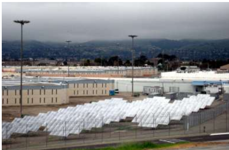
Figure 3: Recent photo of Santa Rita jail with ground mounted tracking solar PV in foreground and batteries and fuel cell directly behind
