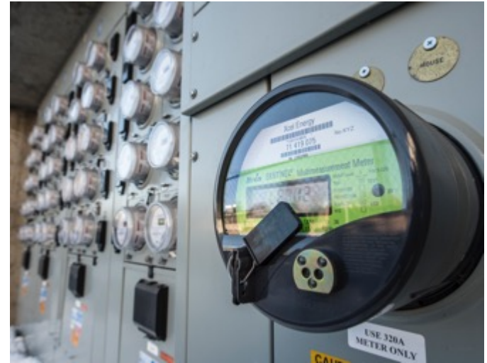
(Photo by Dennis Schroeder / NREL #48963)
