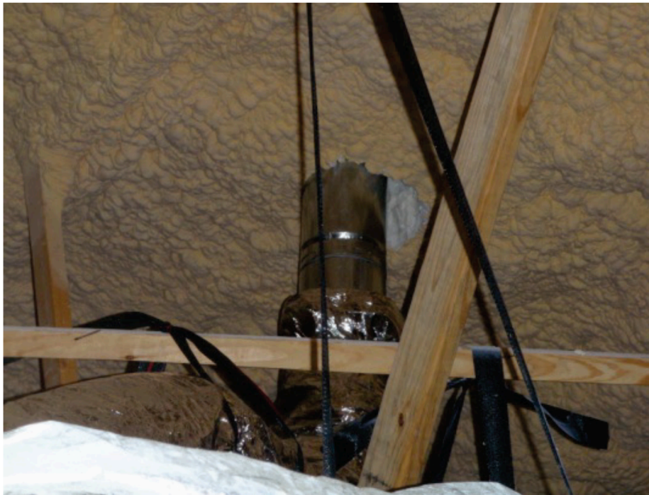
Figure 8 Example picture of gaps surrounding roof vent pipe penetrations. Source: Prahl and Shaffer (2014).
