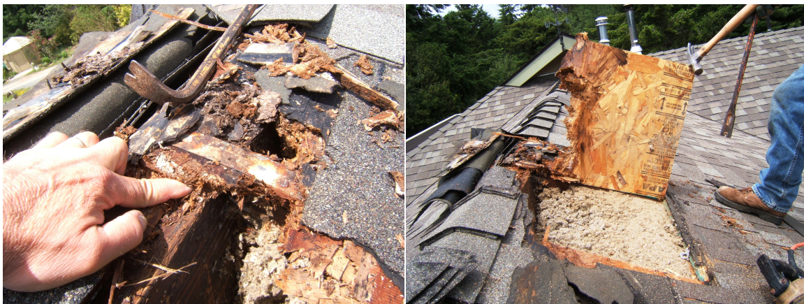
Figure 18 Photographs of deconstruction of a sealed and insulated attic assembly with dense pack cellulose on a home in Northern California that had experienced water dripping at the roof ridge.
