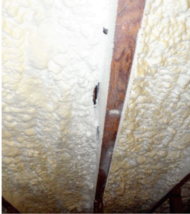
Figure 7 Example image of closed cell SPF delamination from roof framing member. Source: Prahl and Shaffer (2014).
