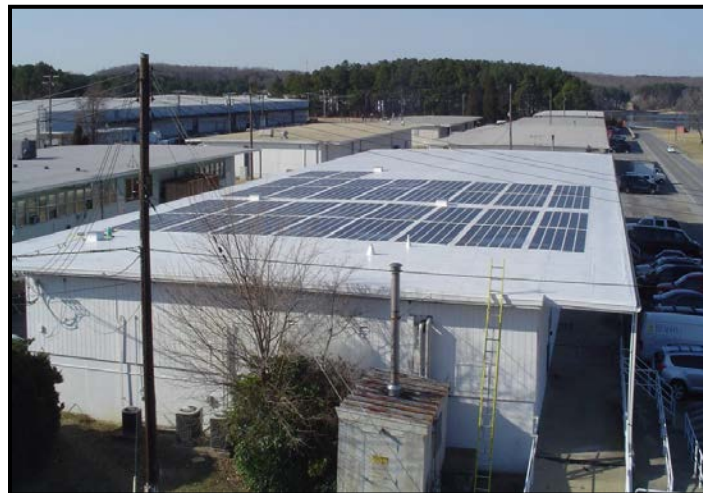
Figure-10: Photo of Building 515 at NAS Patuxent River after BIPV installation.
