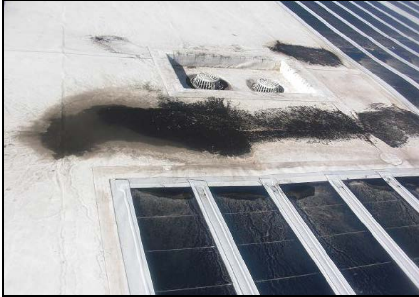
Figure-47: Severe, localized mold growth due to water ponding before it reaches the drains.
