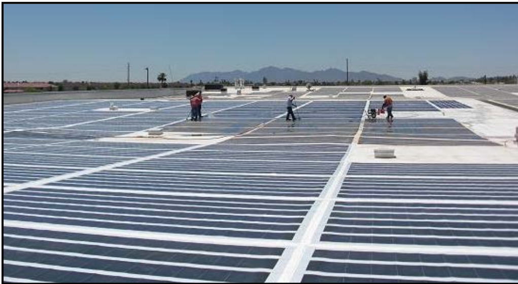
Figure-8: Luke AFB BIPV roof being cleaned during adhesive-failure fix.
