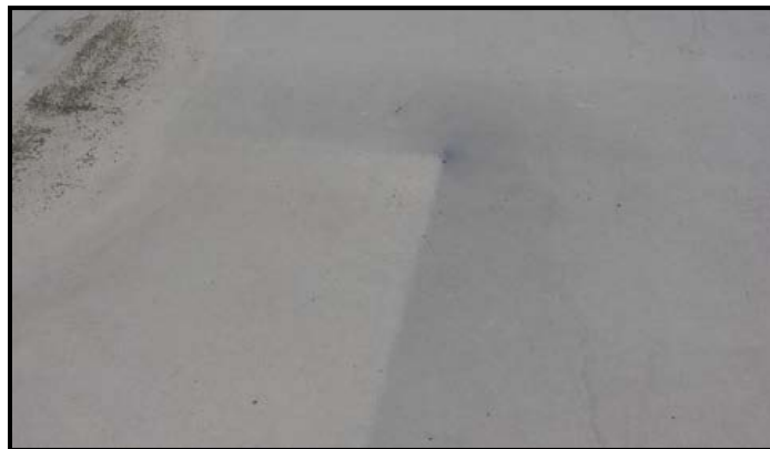
Figure-28: Mold growth (upper left corner) and warping dens-deck (center) at Site II (NAS Patuxent River).
