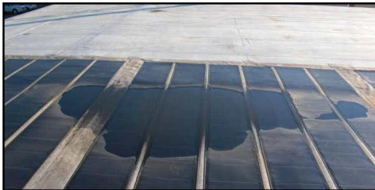
Figure-29: Significant ponding at Site II (NAS Patuxent River).
