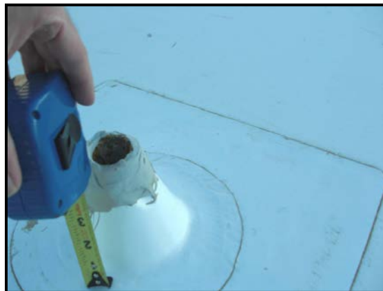
Figure-44: Photo of Site III (MCAS Yuma) air vent with insufficient flashing height.
