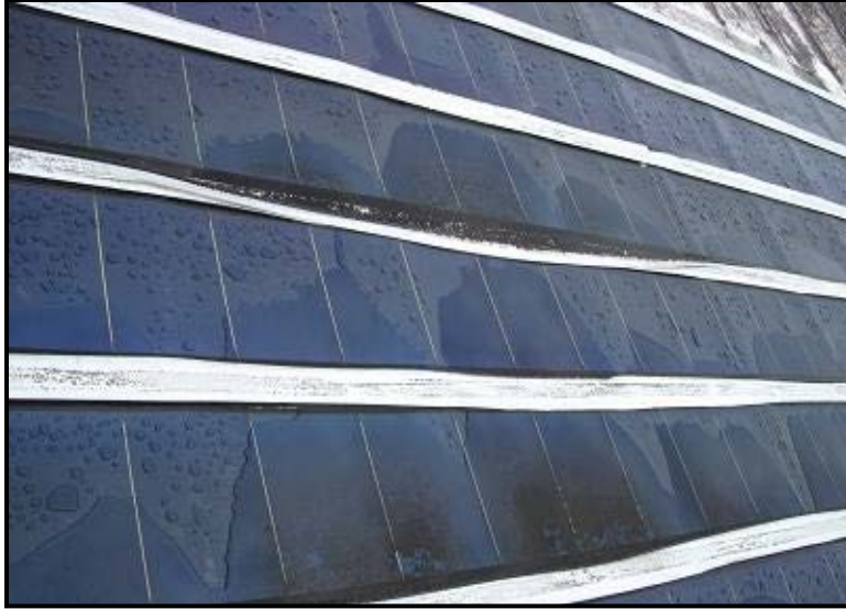
Figure-45: Water ponding due to the failing tape and PV module orientation. Mold growth in the upper right corner.
