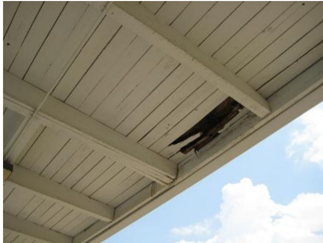
Figure 3 Building 515 Rotten Section
