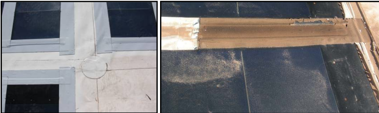
Figure-21: Tape solution soon after it was applied (left) and deterioration later that year (right) Site I (Luke AFB).
