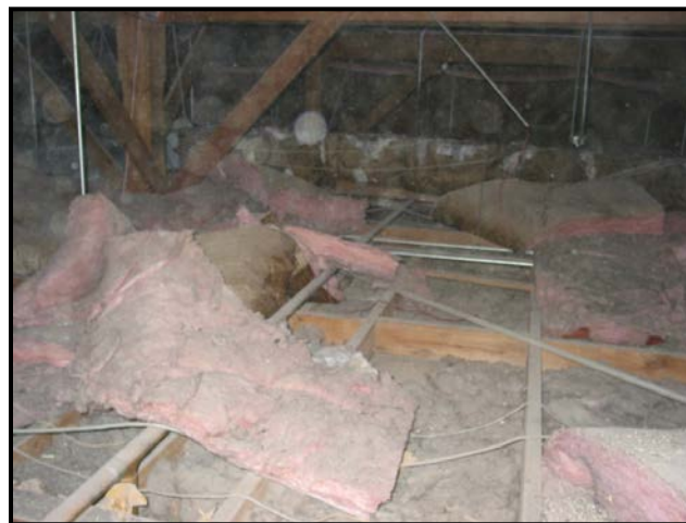
Figure-12: Attic space of Building 228 at Site III (MCAS Yuma) showing poor insulation.
