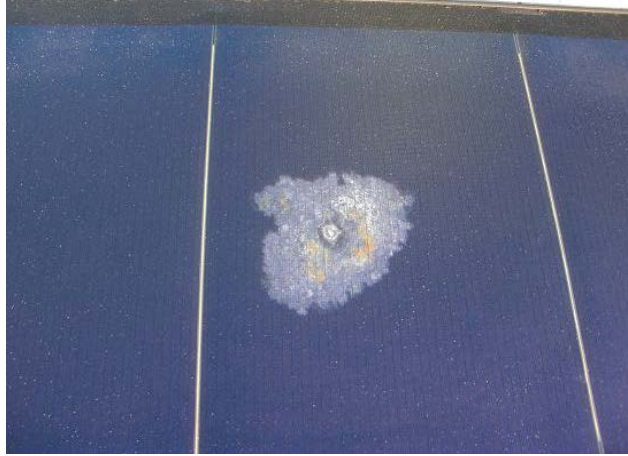
Figure-50: Corrosion of PV material due to a pin-size hole at Site II (NAS Patuxent River).
