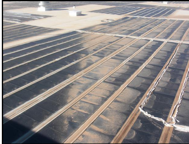
Figure-22: Tape deterioration and soiling of the PV system at Site I (Luke AFB).
