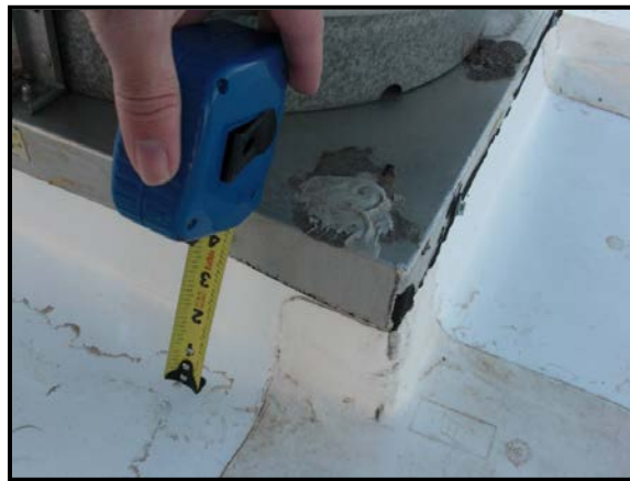
Figure-43: Photo of Site III (MCAS Yuma) exhaust vent with insufficient flashing height.
