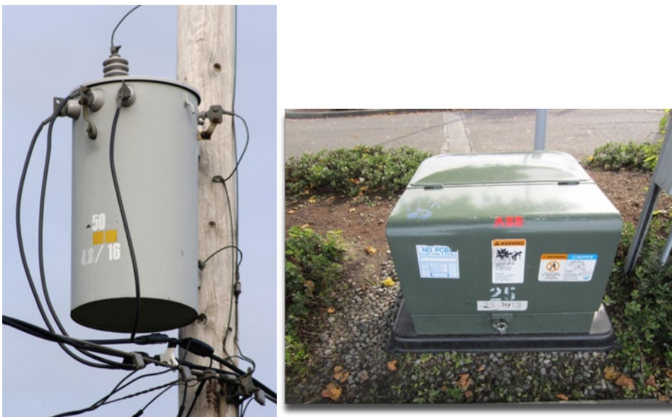
Figure 6. Overhead (left) and padmount (right) service transformers (Source: EPRI)
