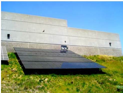
Figure 10. one of two photovoltaic arrays (~6 kW) at the San Diego P&DC
