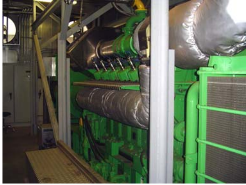
Figure 8. General Electric Jenbacher 1.5 MW reciprocating engine installed at the San Diego P&DC
