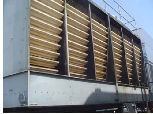
Figure 9. cooling tower for chillers at the San Diego P&DC
