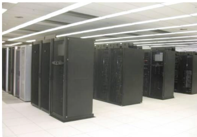
Figure 2-1: Demonstration Data Center IT Equipment
