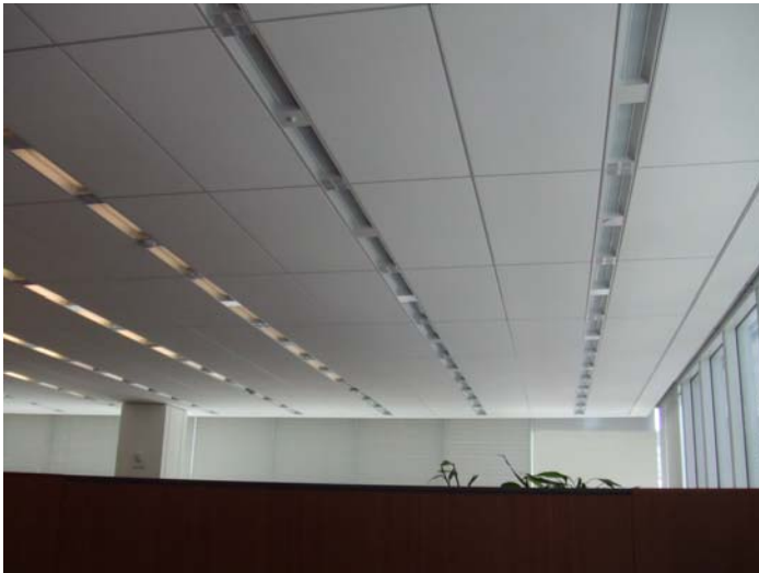
Figure 1-5. View towards the south near noon on a sunny day (8 th floor, shading and lighting commissioned). Note the large number of fixtures that are off due to the large amount of daylight. Note also that many other fixtures are deeply dimmed as well confirming that the lighting system is performing as expected.
