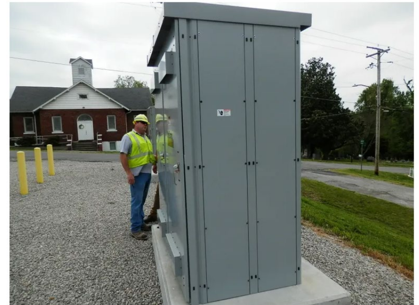
Ameren Illinois Thebes Battery [ Link ]
