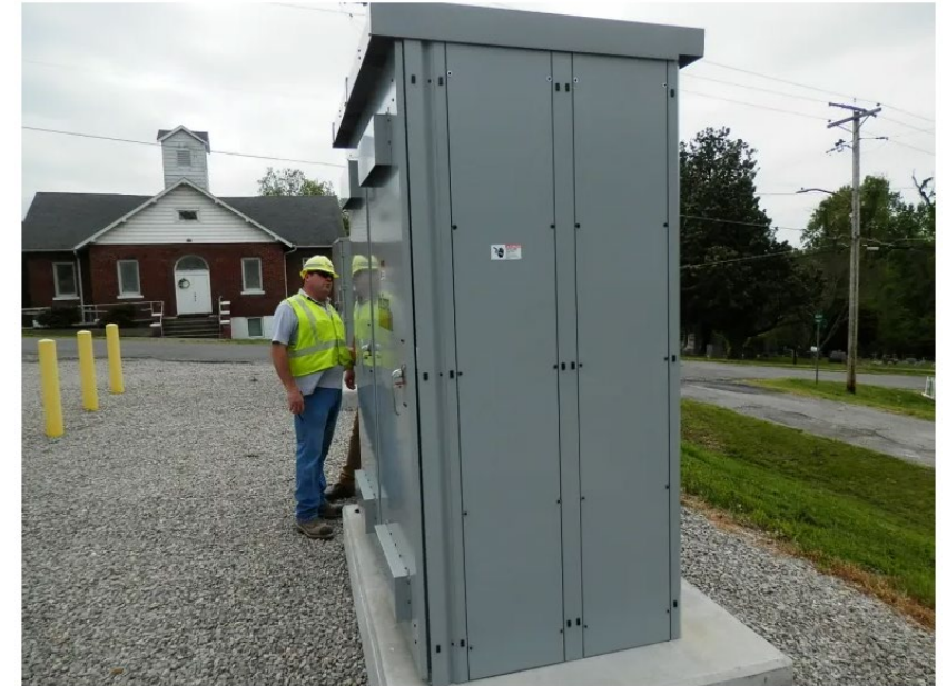
Ameren Illinois Thebes Battery [ Link ]
