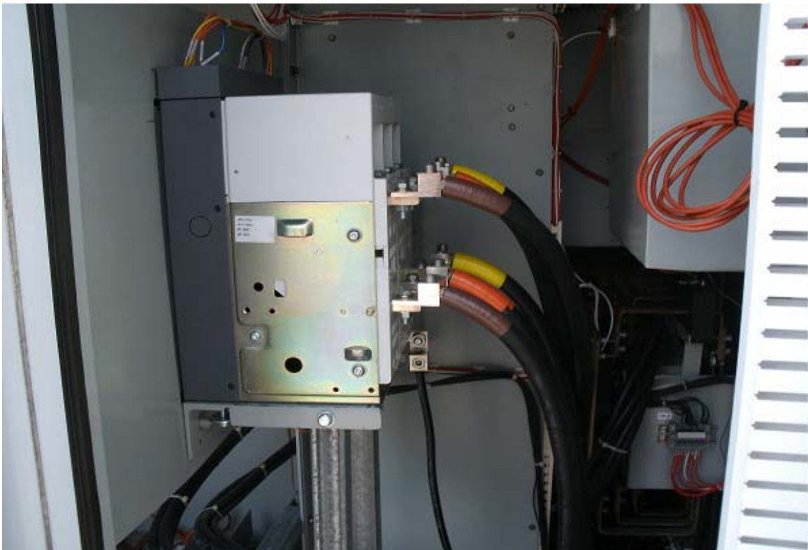
Figure 13: Rear view of MS17 in static switch cabinet
