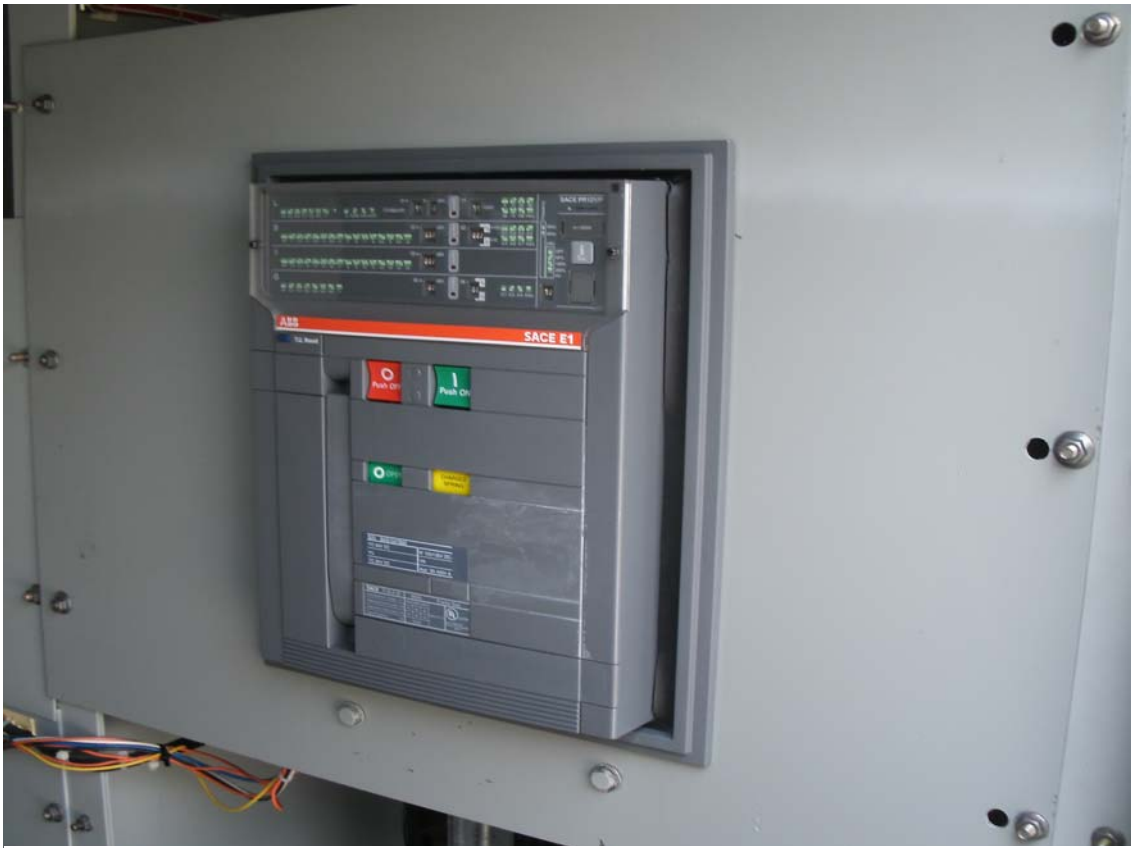
Figure 12: Front view of MS17 in static switch cabinet
