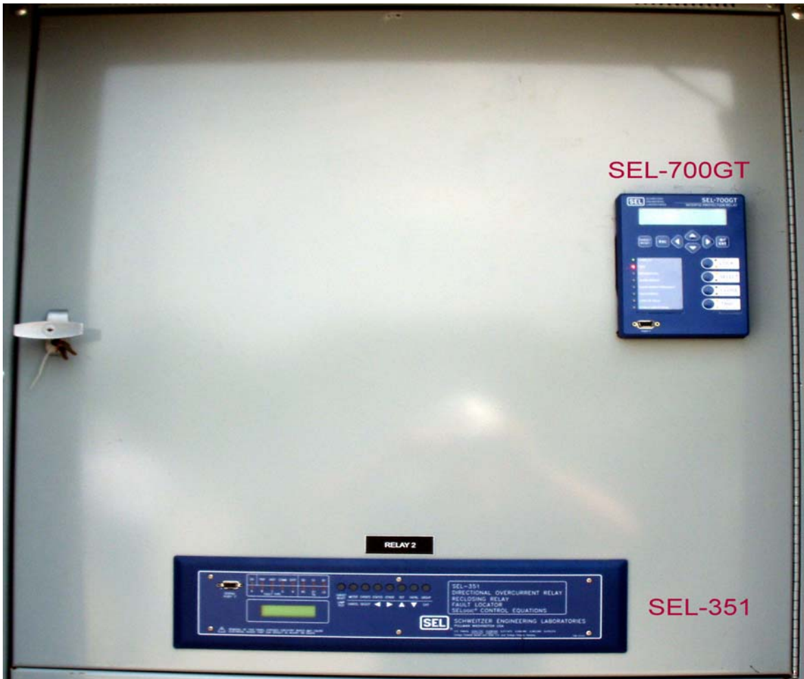
Figure 10: Front panel of SEL-700GT and SEL-351 in cabinet 2a
