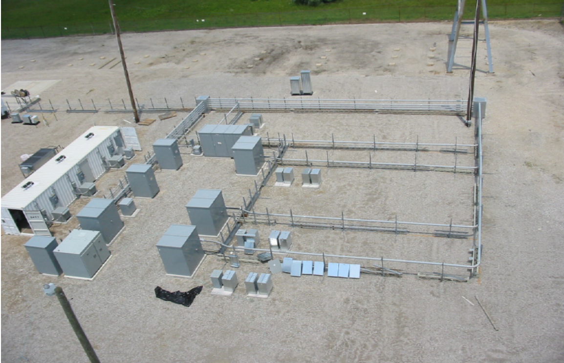
Figure 1 - CERTS Microgrid Aerial Photo
