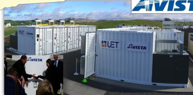
1 MW / 3.2 MWh UET vanadium-flow battery – Pullman, WA
