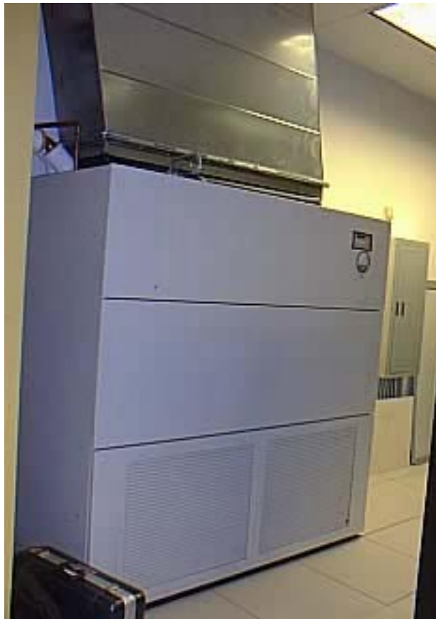
Figure – Data Center Air Handling Unit
