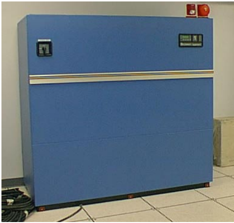
Data Center CRAC Unit
