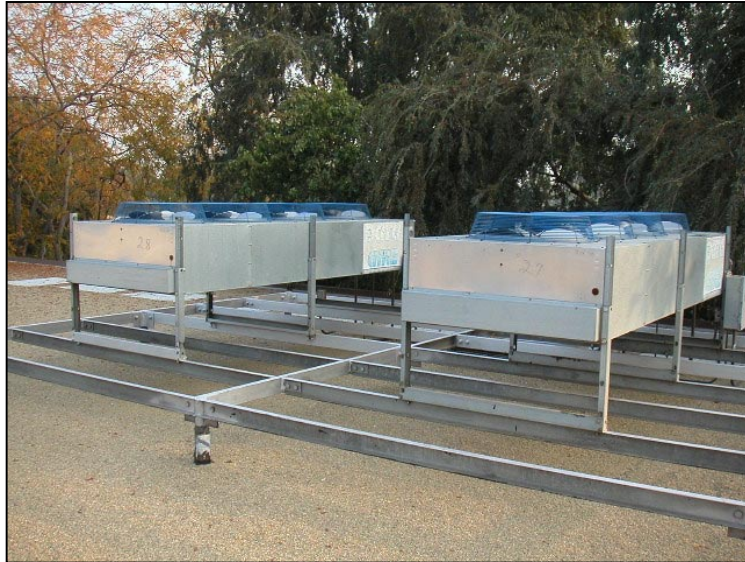
Figure 12. Air-Cooled Condensers on Roof
