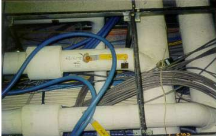
Figure 13 This under floor area severely restricts air flow
