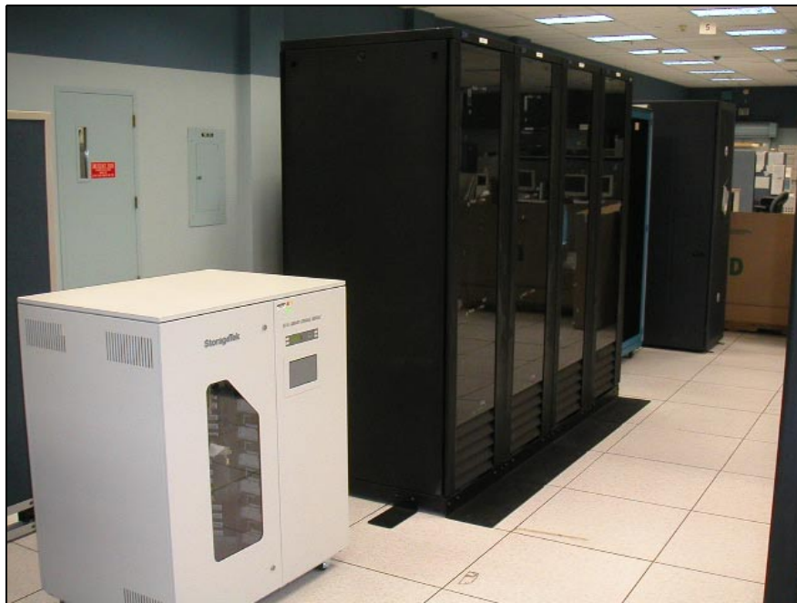
Figure 11. Servers in Data Center 4.5
