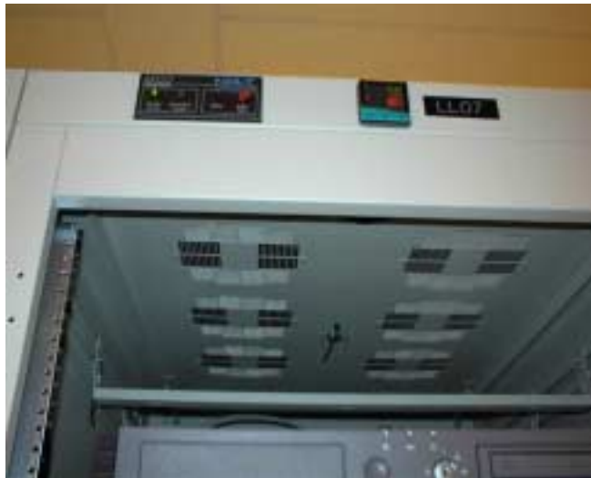
Figure 7 Top of cabinet showing fans
