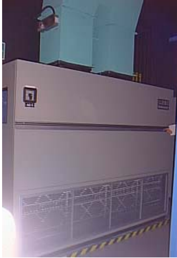
FIGURE 2. DATA CENTER CRAC UNIT
