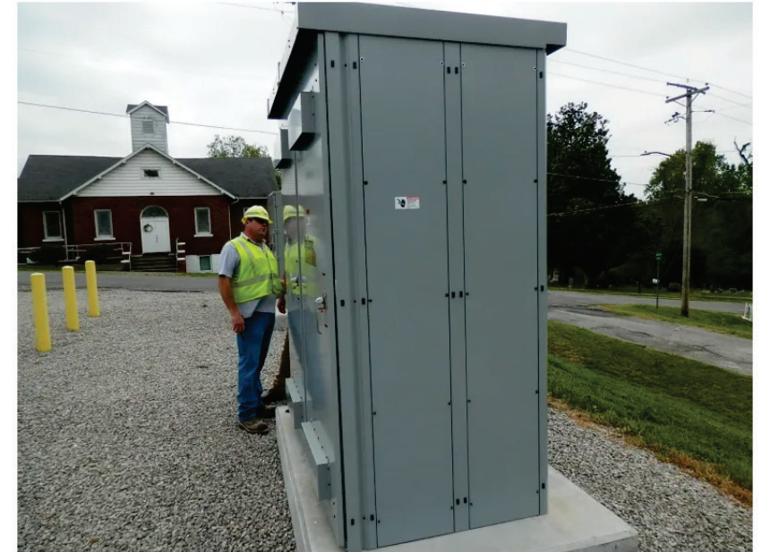
Ameren Illinois Thebes Battery [ Link ]
