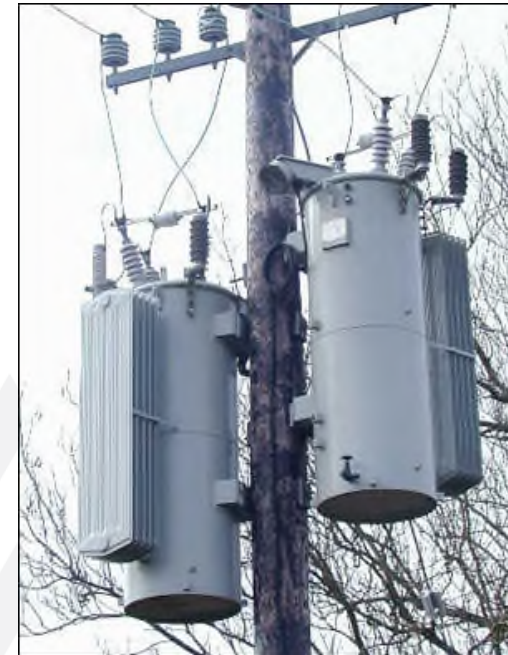
2 Single Phase Voltage Regulators
