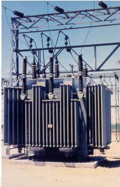
Substation transformer with load tap changer
